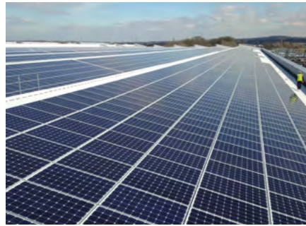
Solar array at our Engine Manufacturing Centre (EMC) at Wolverhampton.
